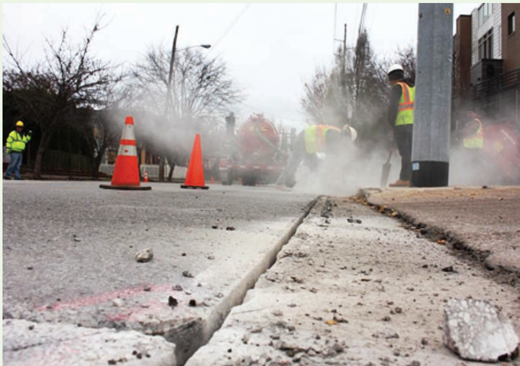
An example of Urban Disruption caused by trenching. Credit: WPLN/Tony Gonzalez.
