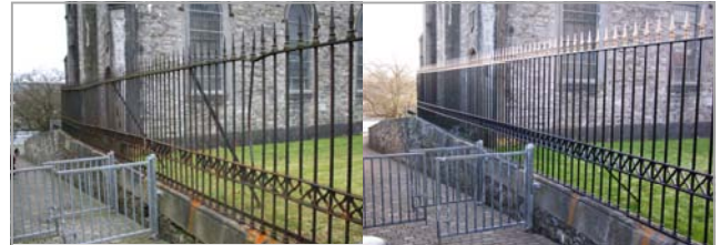
The railings at Calry Parish Church, The Mall, Sligo before and after works completed.
