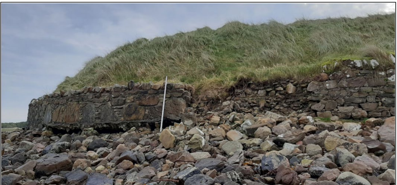
Figure 1.3: Kilaspugbone Graveyard – undermining incl. collapse of a short stretch of wall (Sligo County Council, 2021)
