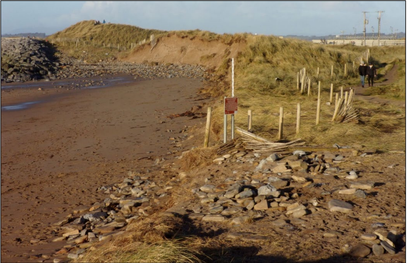
Figure 1.2: Dune erosion and area of sea ingress into dunes south of rock revetment at WWTP (Sligo County Council, 2021)
