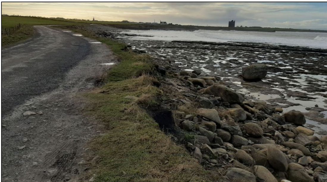
Figure 6.3: The road near Easkey Castle indicating erosion/ damage (Sligo County Council, 2021)
