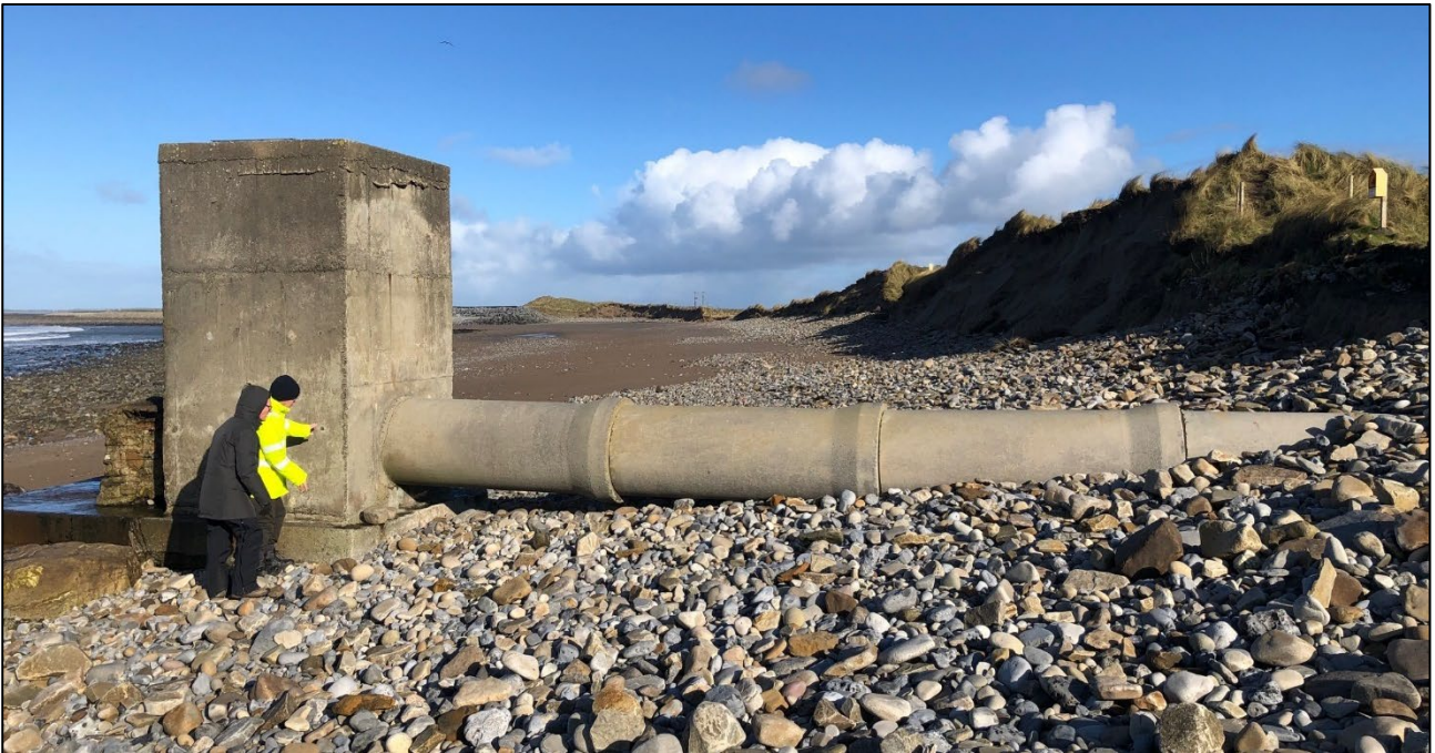
Figure 4.7: Exposed storm water manhole north of Strandhill, February 2022
