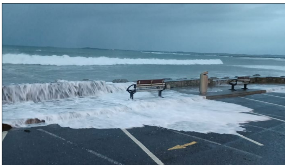
Figure 5.2: Wave overtopping of the rock armour revetment at Strandhill town in February 2022
