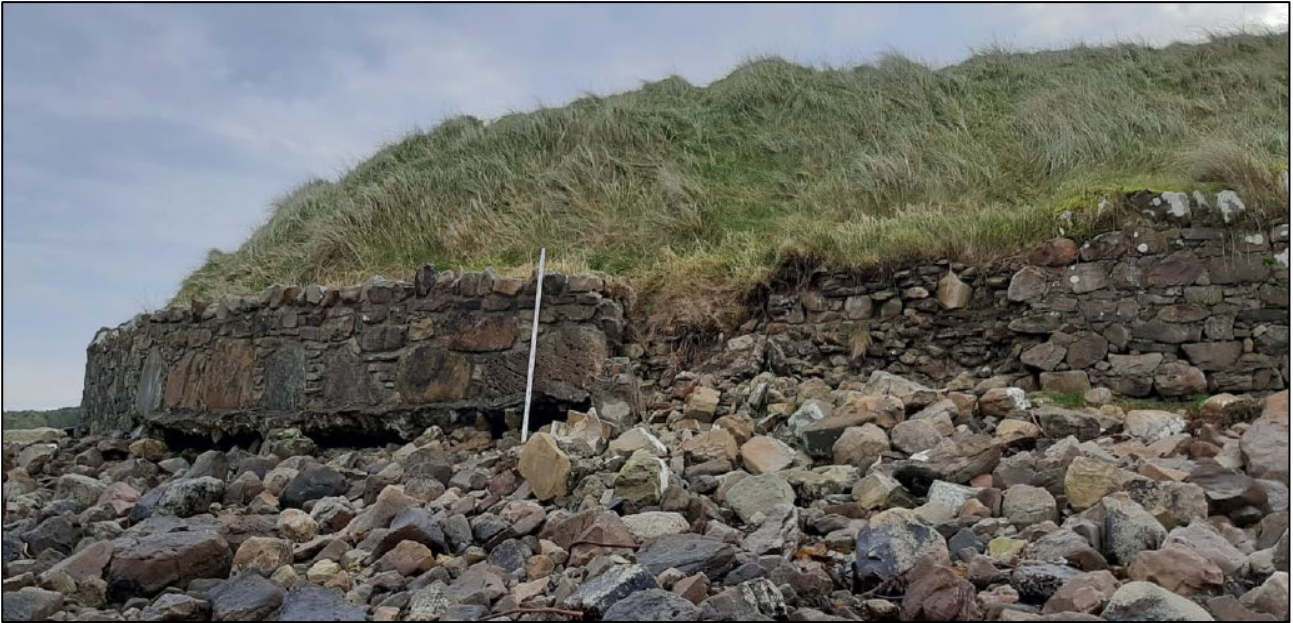
Figure 6.6: Failure of the informal coastal defence at Kilasprugbone Graveyard
