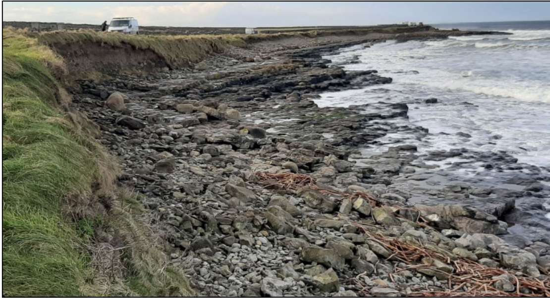
Figure 6.2: A section of the road showing signs of coastal erosion (Sligo County Council, 2021)
