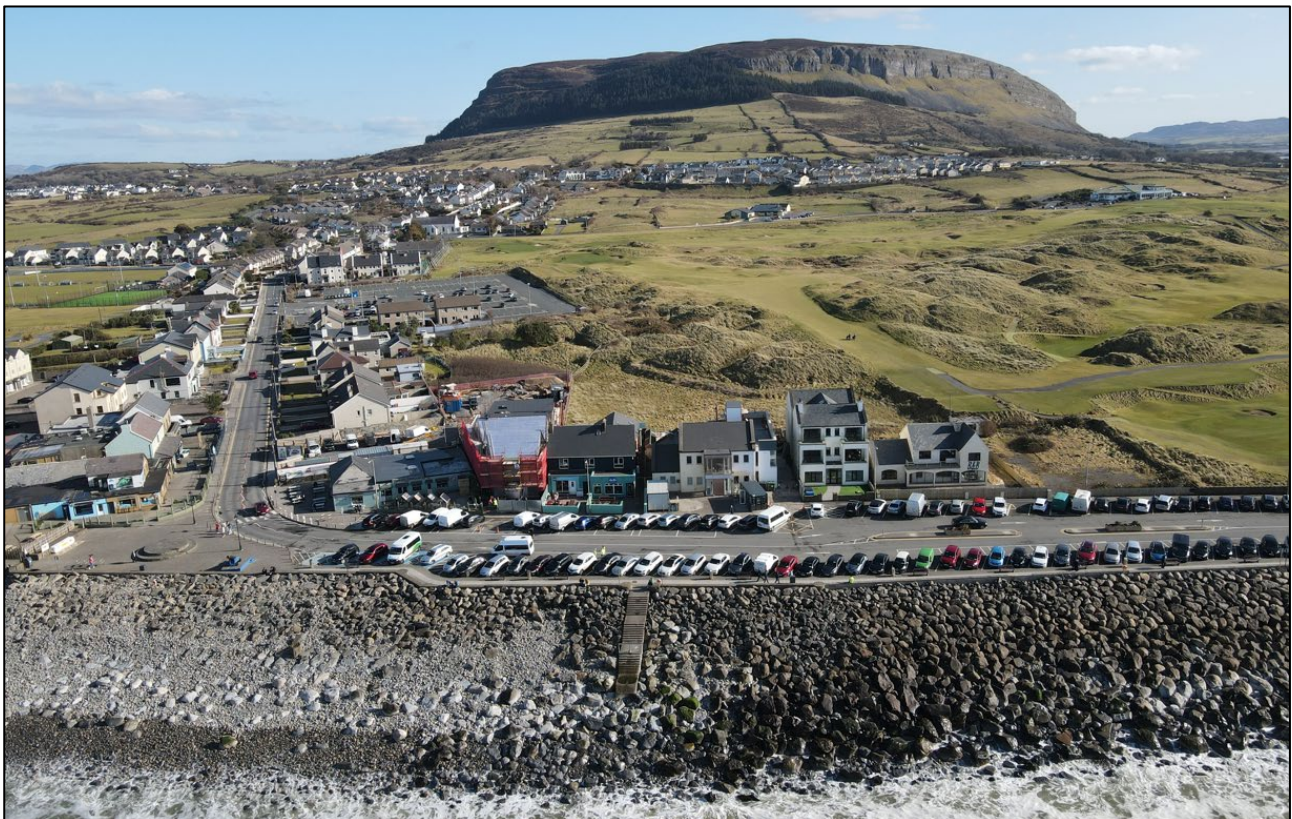
Figure 6.5: Poor condition of northern rock revetment (left) compared to the well-maintained southern section (right)
