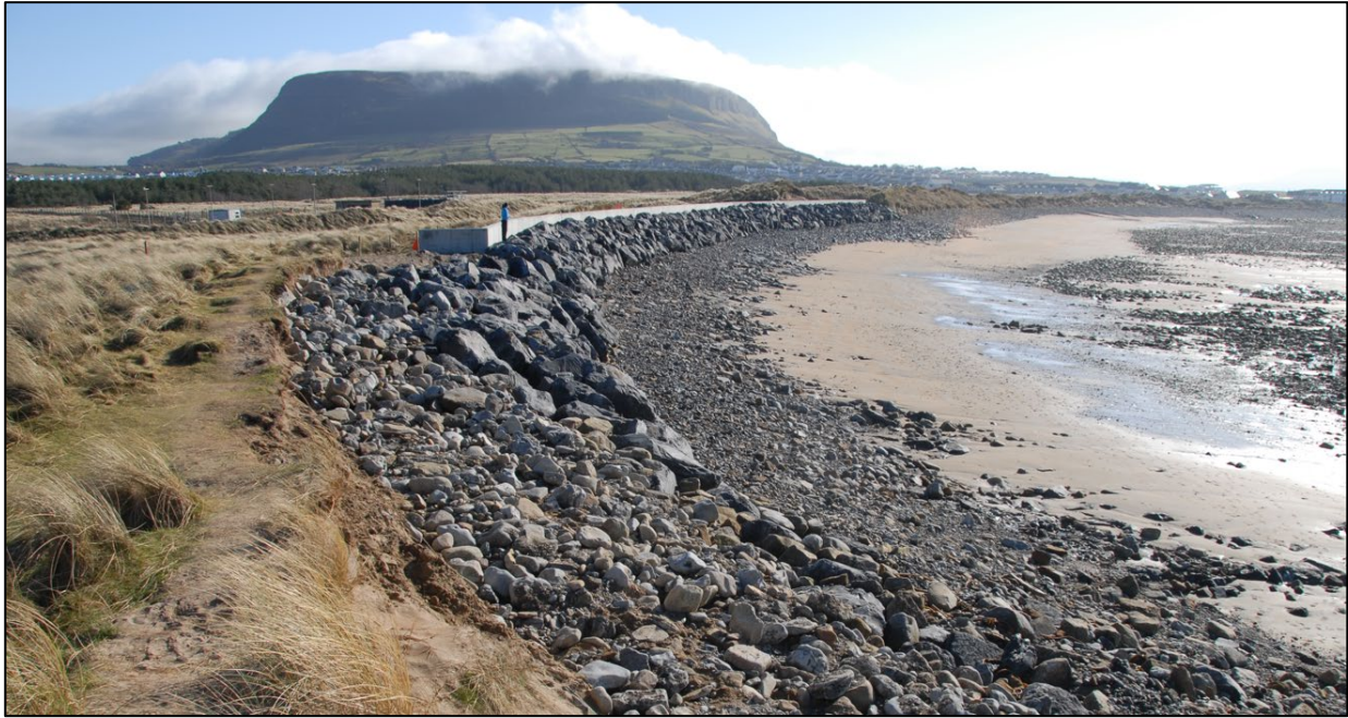
Figure 4.5: The coastal protection works at the Wastewater treatment works following construction in Feb 2011
